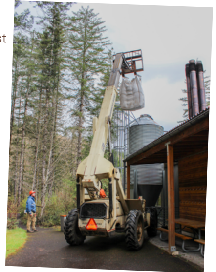
Wood pellets being delivered into the silo for our boilers.
