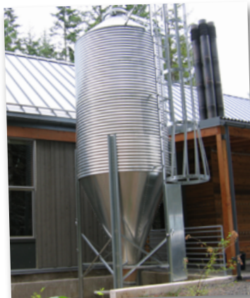
The wood pellet silo holds 12 tons or enough pellets to heat the building for about three months.
